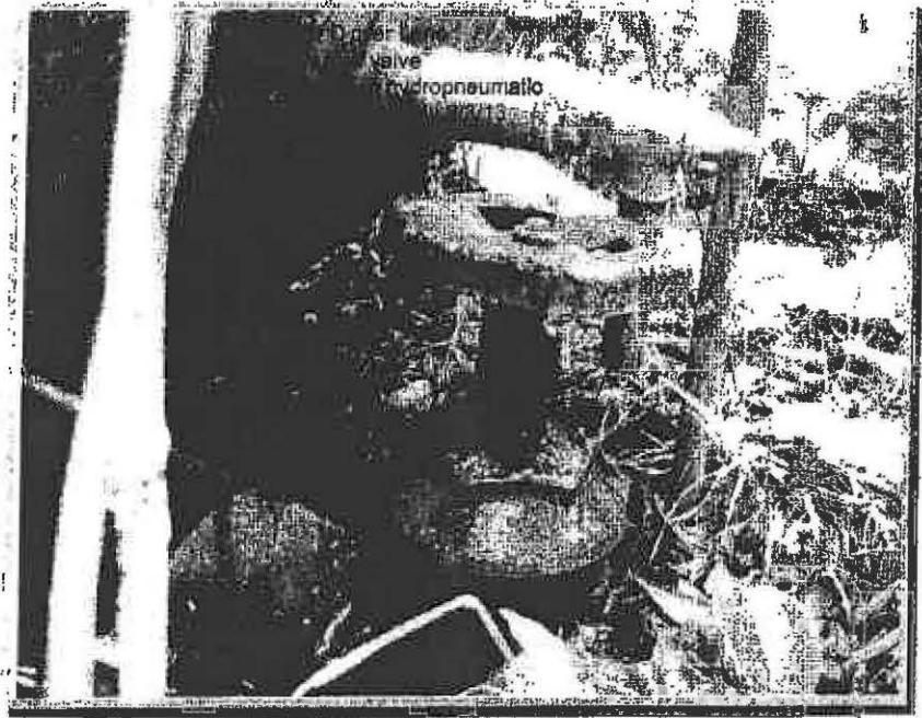
Failed (leaking) Valve
